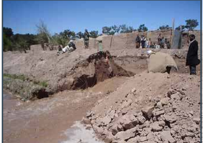
Illustration 7: Breach in main canal (April 2005)
