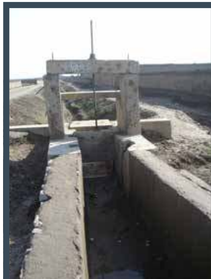
Illustration 23: Tertiary control gate, Parwan scheme (Bob Rout photograph)
